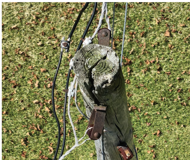
EYE IN THE SKY: This drone image shows a pole with a split top, which causes weak connection points and contributes to the pole's decay.
